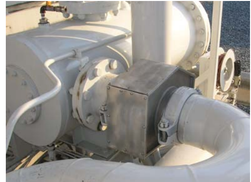
VCA in Operation at Dubai International Airport
